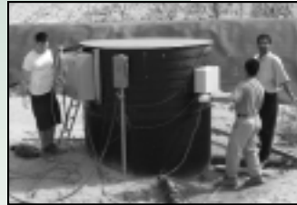
Leachate sump and monitoring equipment is routinely tested and inspected.
